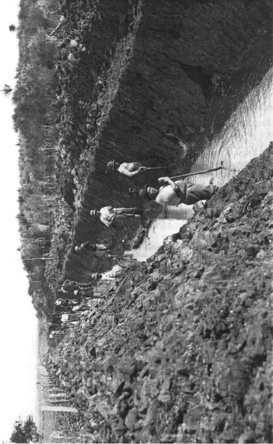
Draining the Kaitaia swamp early this century. From the Northwood collection, photograph courtesy of the Alexander Turnbull Library (G10661 1/4).
